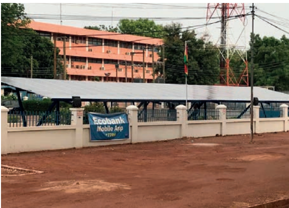
Ecobank Ghana: Solar panels at the Tamale branch
