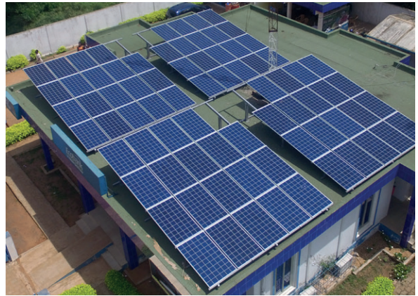
Ecobank Togo: Solar panels at the University branch
