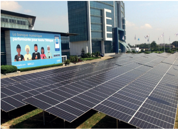
Togo: Solar panels at Ecobank's Pan African Centre
