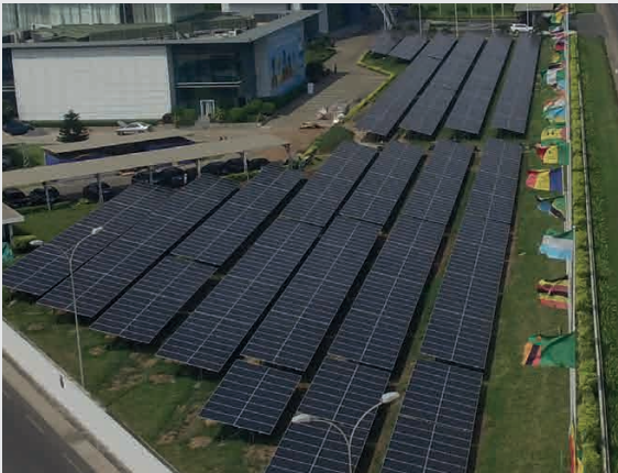
Solar panels, Ecobank Togo
