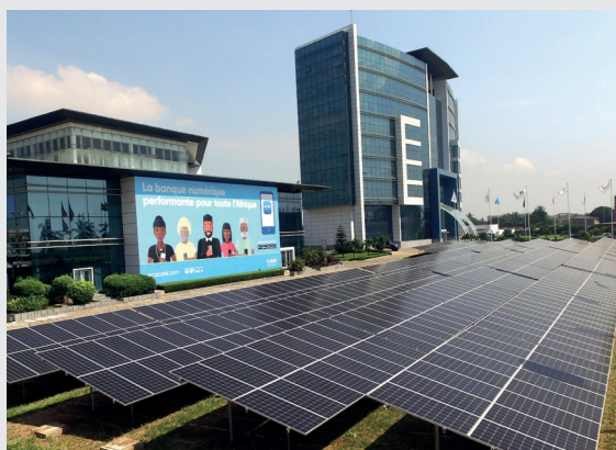
Solar panels, Ecobank Togo
